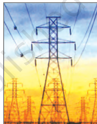
Fig. 3.7: National Power Grid to supply Electricity
